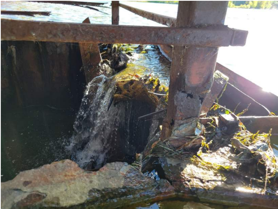
Photo 3: Rotted Post Supports
