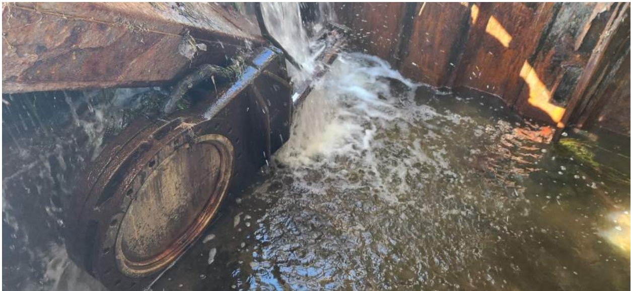
Photo 8: Knife Gate & Broken Sheet Pile Cap
