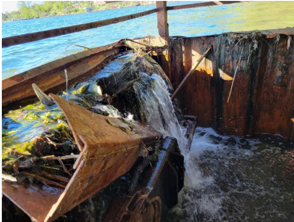
Photo 9: Debris Skimmer & Sheet Pile Cap
