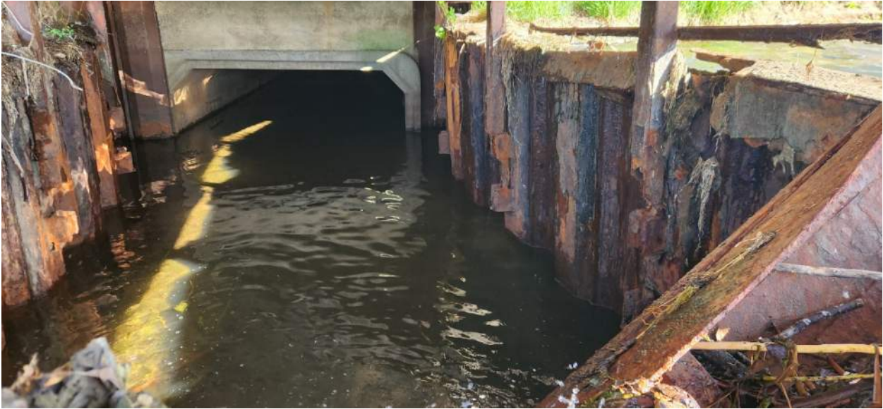
Photo 5: Rotted Post Supports
