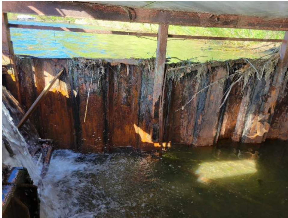
Photo 2: Rotted Post Supports
