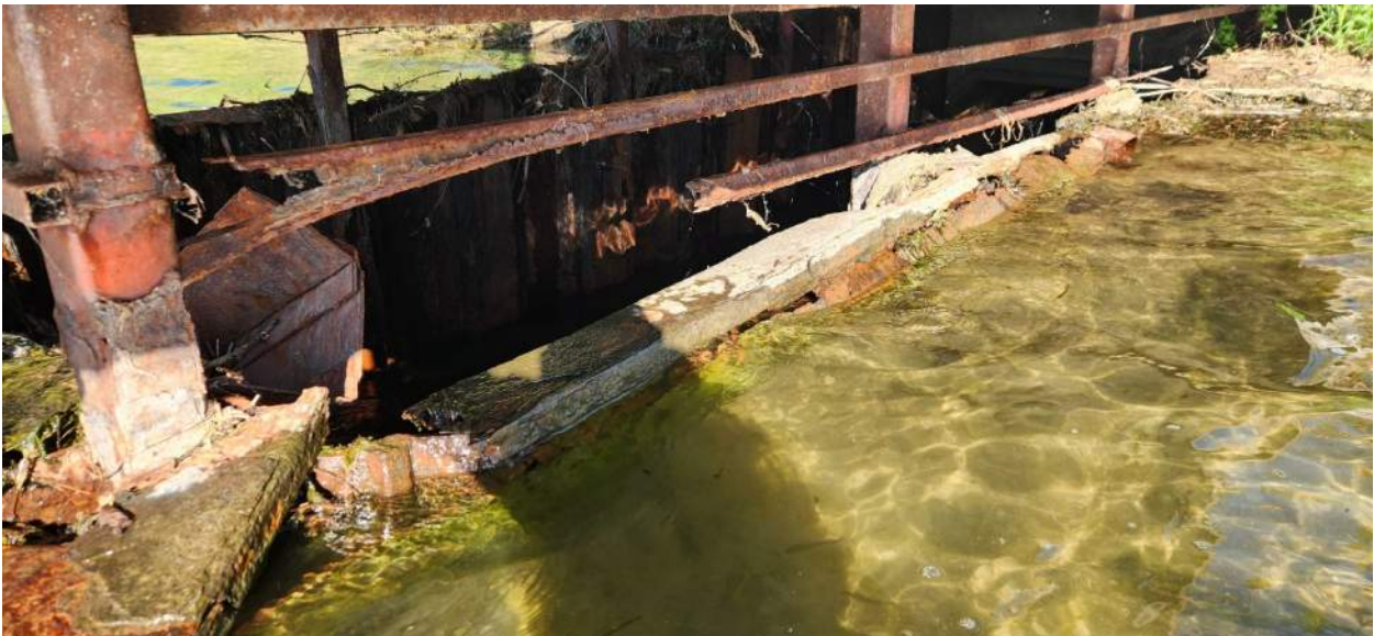
Photo 6: Broken Underside Railing
