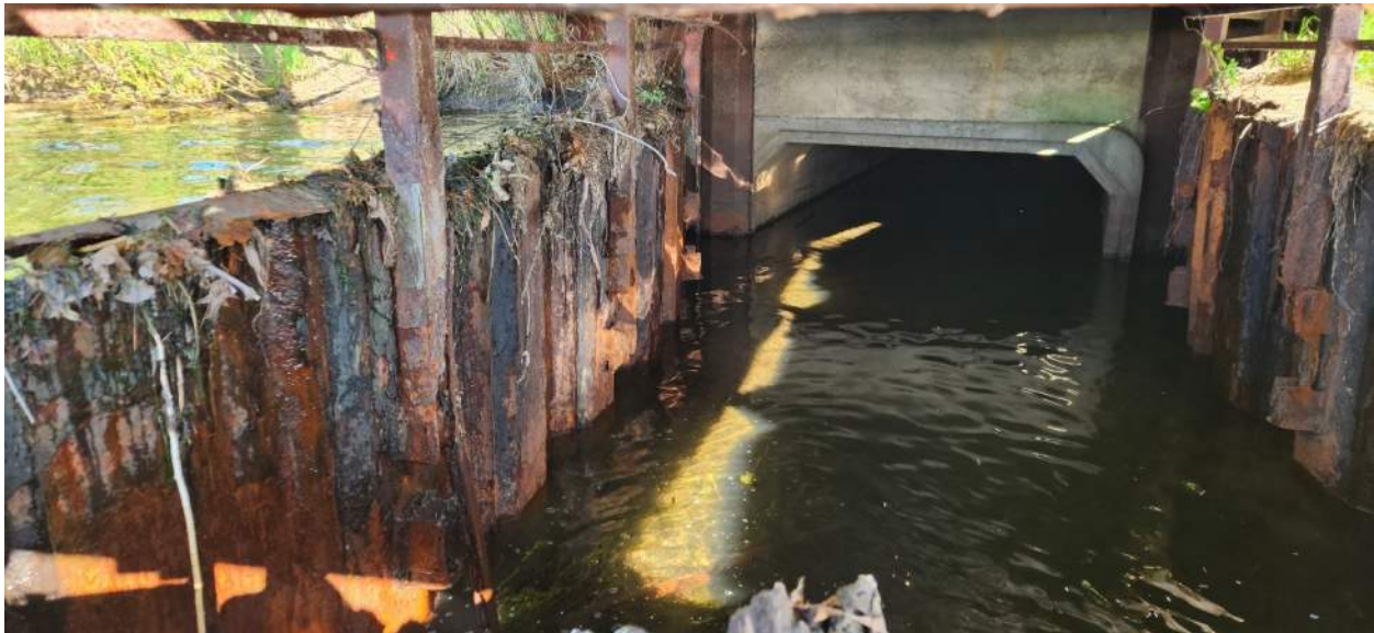
Photo 4: Rotted Post Supports
