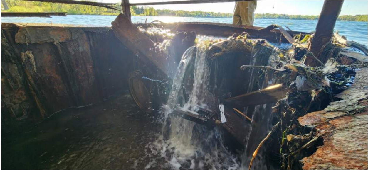
Photo 7: Knife Gate & Broken Sheet Pile Cap
