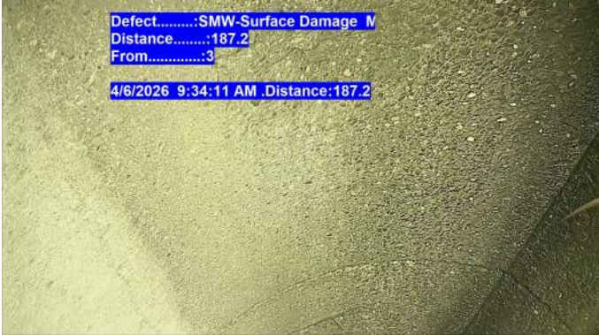
Img:3,Distance:187.2 Surface Damage Missing Wall,@:3,Rmk:
