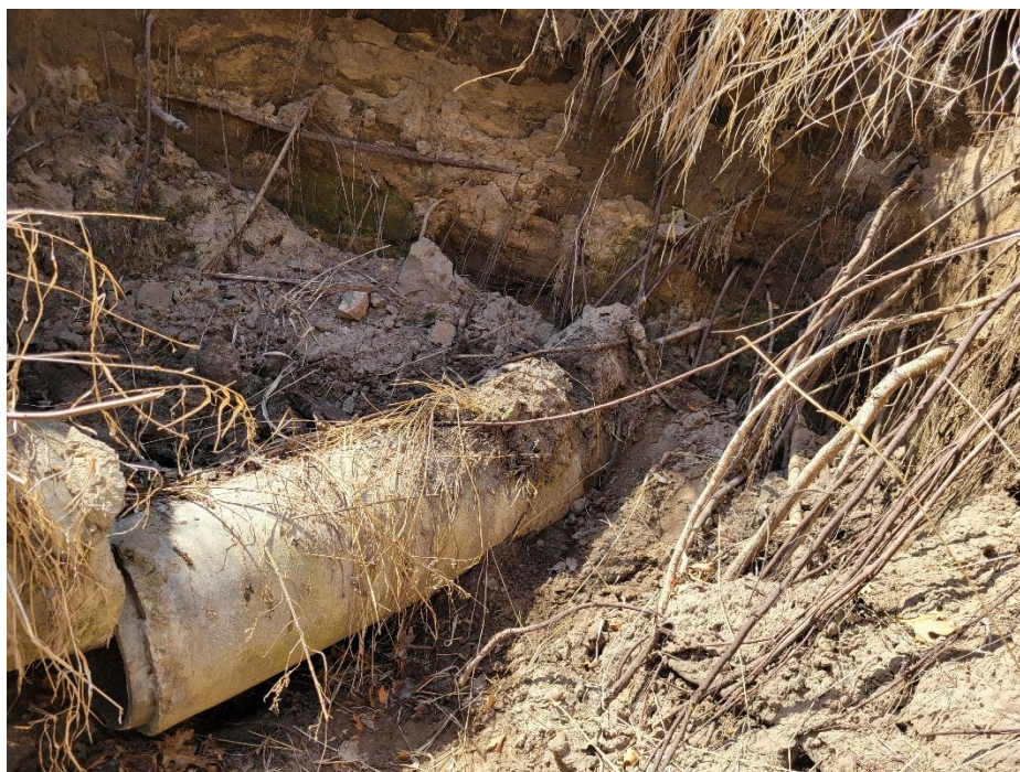
Photo 4- Dislodged pipe segments
