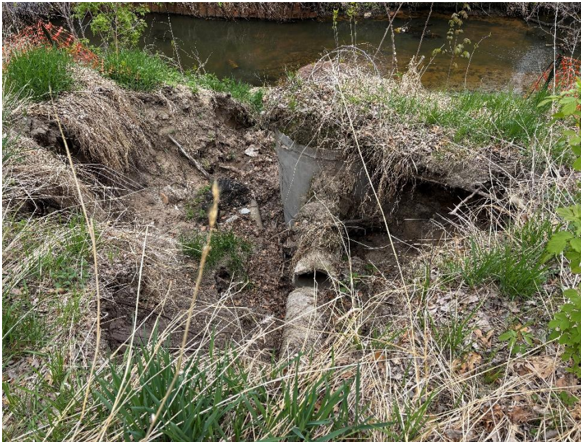
Figure 1. Stormwater Outfall Failure
