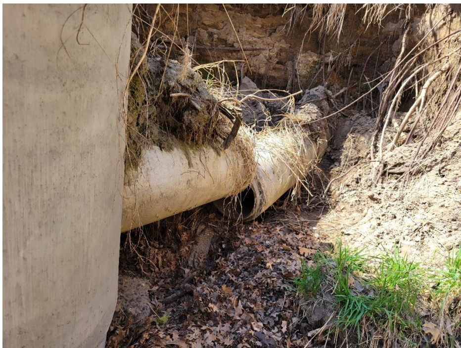
Photo 3- Dislodged pipe. Note intact pipe segment connected to new structure.
