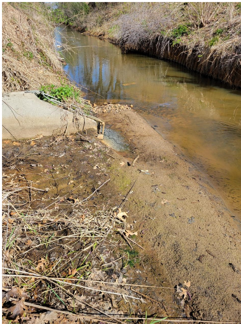
Photo 5- Pipe apron sediment. Note plume of sediment on left side of ditch.
