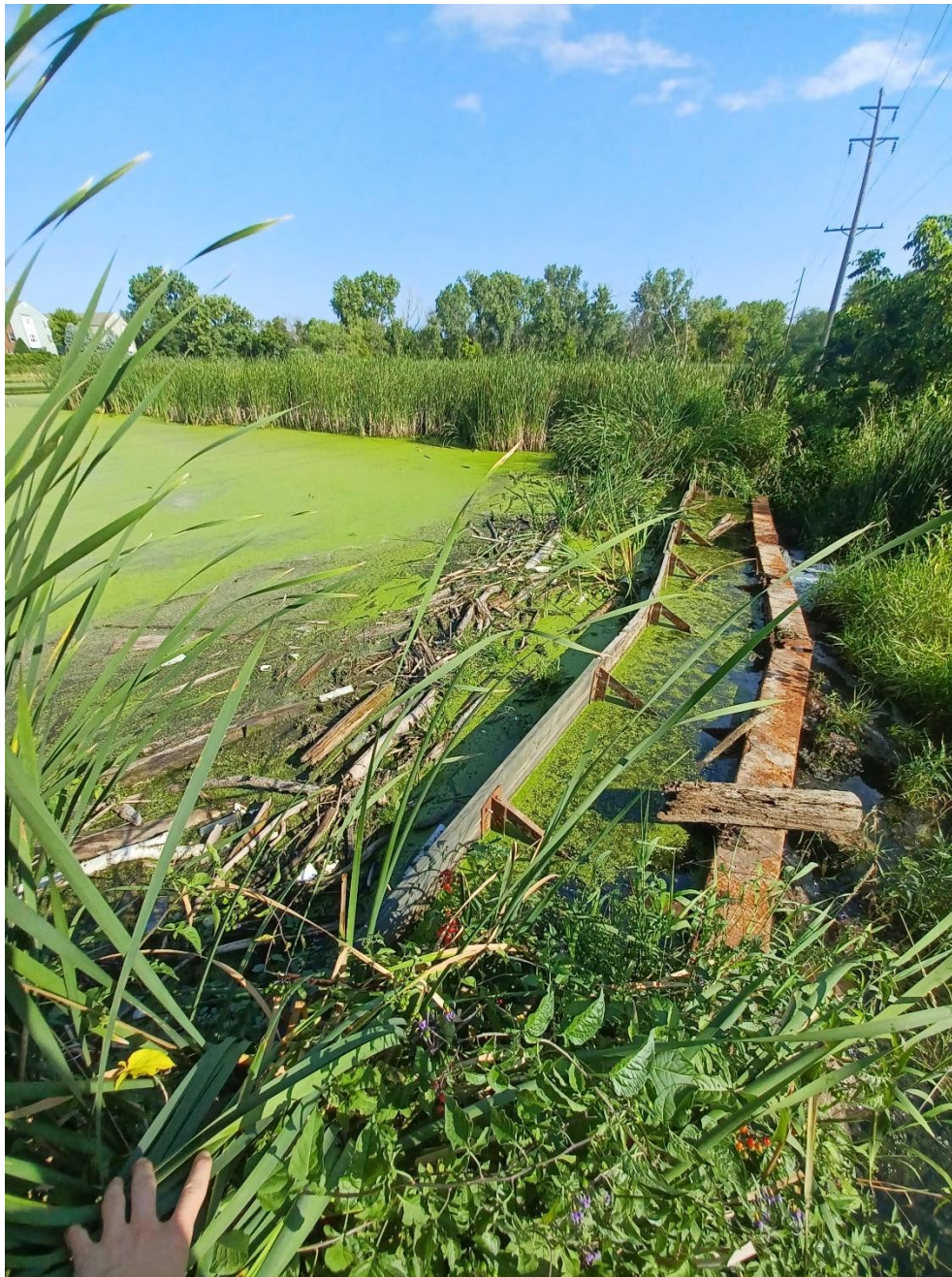
Photo #1: Floating tree debris piled behind weir at STA 5+00
