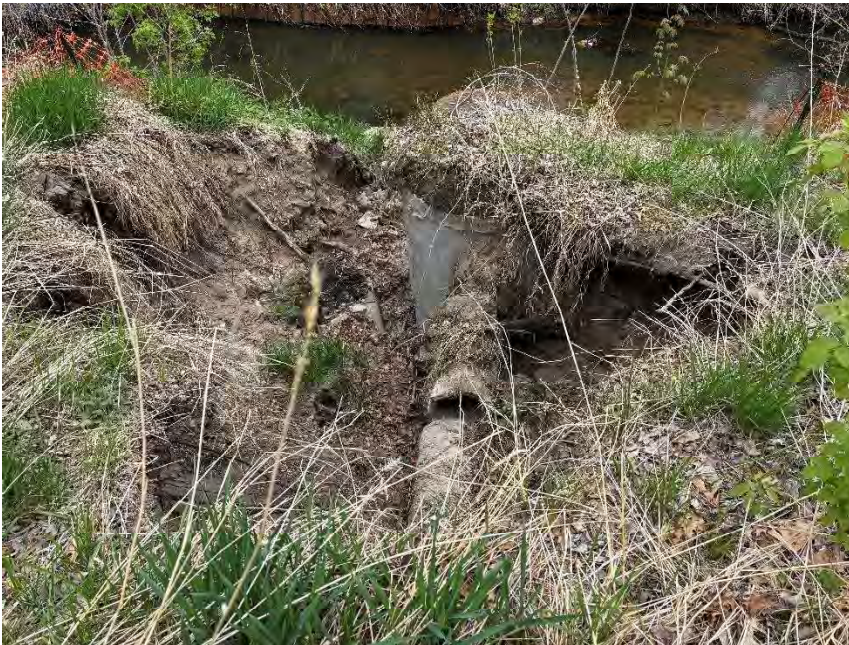
Figure 1. Stormwater Outfall Failure
