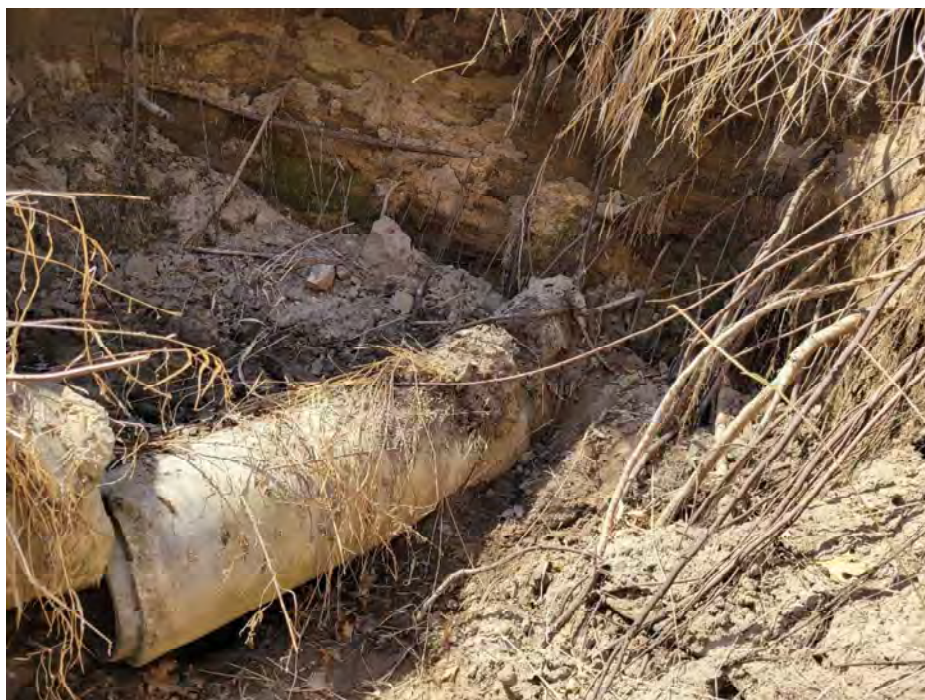
Photo 4- Dislodged pipe segments
