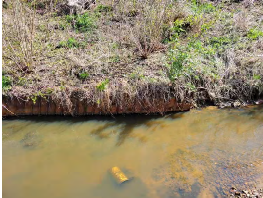
Photo 6- Bank Conditions Across from Pipe Outlet
