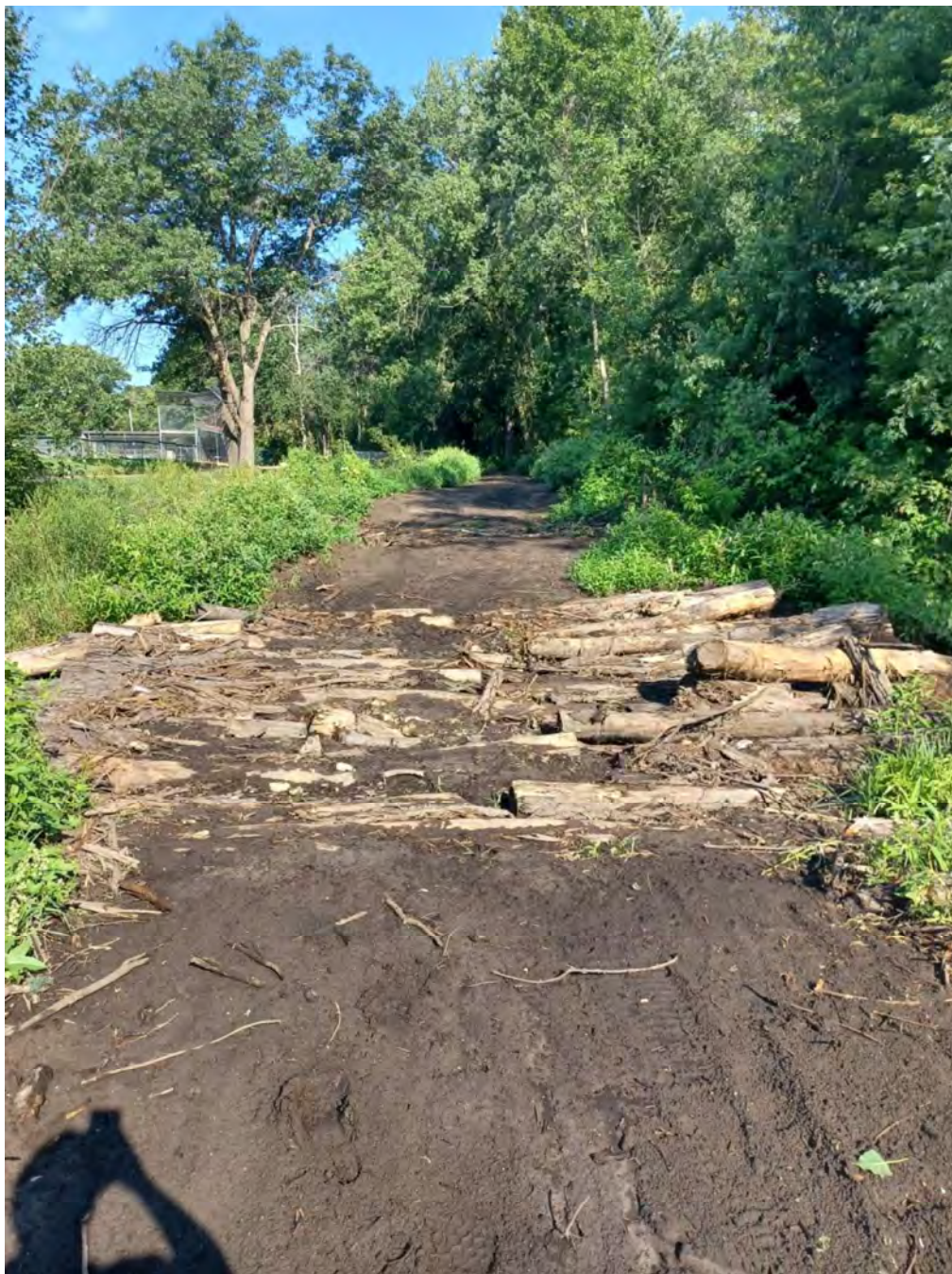
Photo #4: Logs still needing removal near STA 27+00
