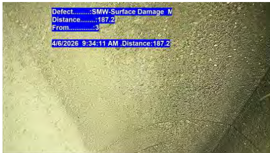
Img:3,Distance:187.2 Surface Damage Missing Wall,@:3,Rmk:
