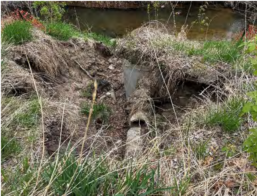
Figure 1. Stormwater Outfall Failure
