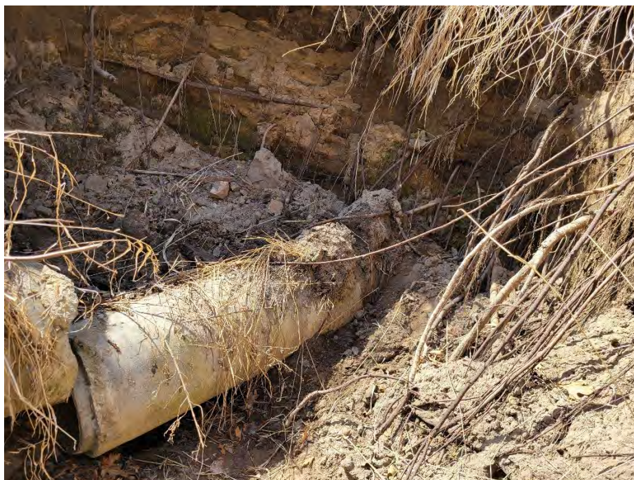
Photo 4- Dislodged pipe segments
