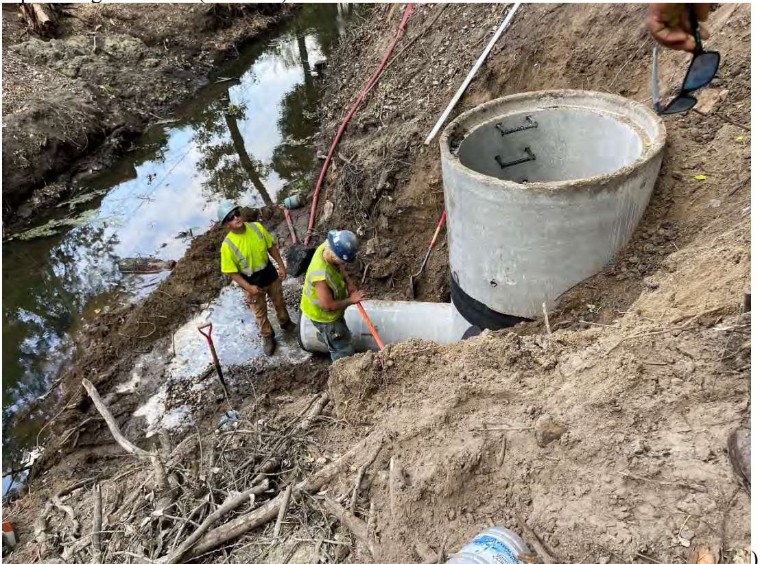
37. Pipe with gasket on it (4:00 PM).
