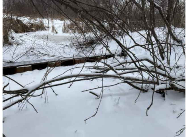
Photo #3: Sheet pile weir with 2x12 board on top, Main Trunk STA: 116+58
